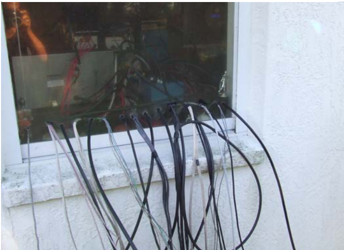
The feedlines and control cables that make it all work at K1TO
