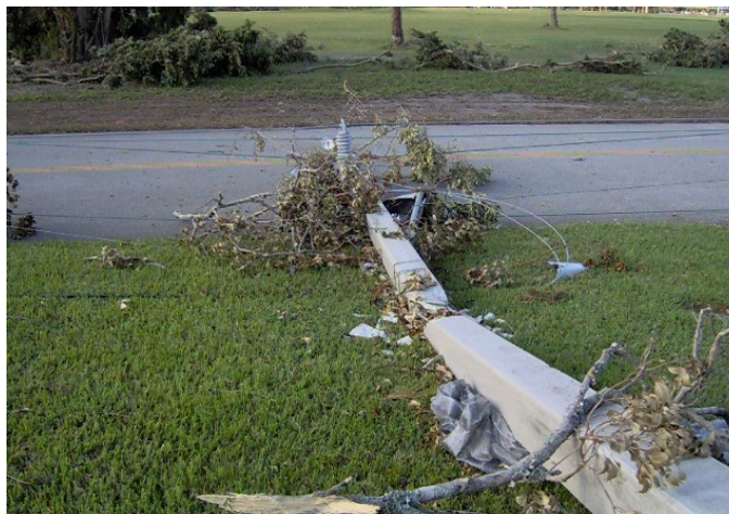
12X12 Concrete Power Pole near W4OV Up since 1967
