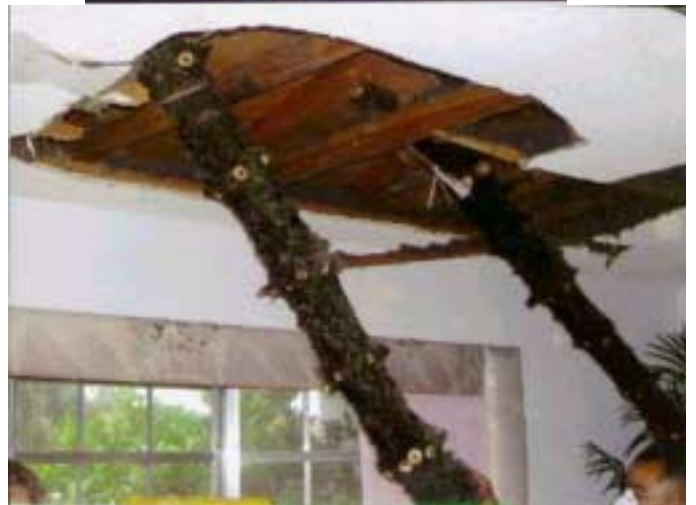
During Frances a 30 ft 800 lb section of a Norfolk Island Pine in front of W4OV's QTH in Coconut Creek broke off and came through his living room ceiling. Tnx Bruce for the pictures.
